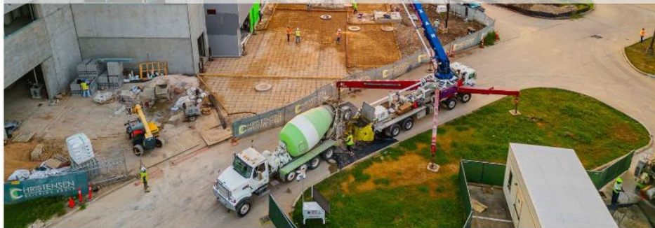
OPUS SCM concrete for the Porsche Sugar Land pour batched, placed, and finished like conventional mixes.
